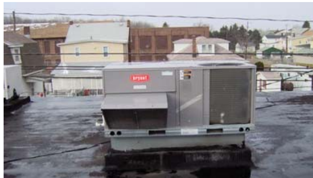
Example of Economizer
